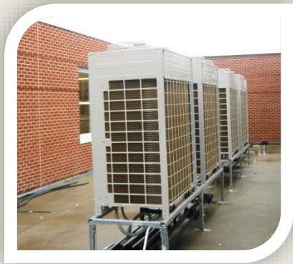
Variable Refrigerant Flow
