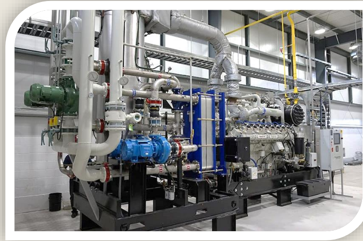
Combined Heat and Power
