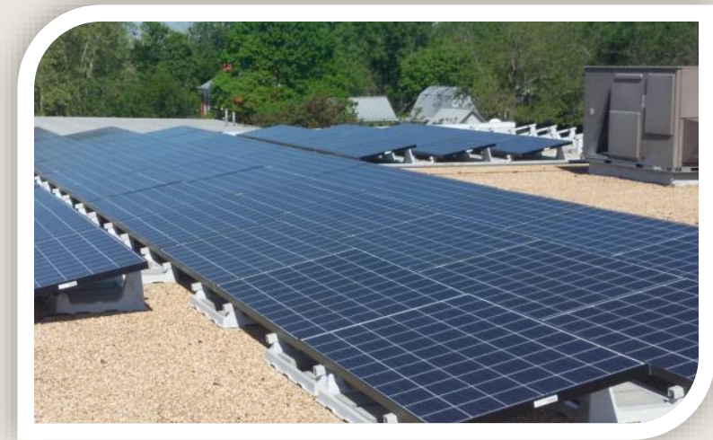
Solar Photo Voltaic Systems
